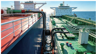
船对船输油管 GS86212-STS Ship-to-Ship Loading GS86212-STS
